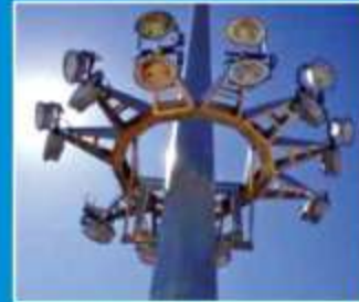
HIGH MAST LIGHT
